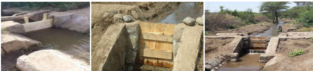
Figure 16: Wooden gates installed on the division box structures
